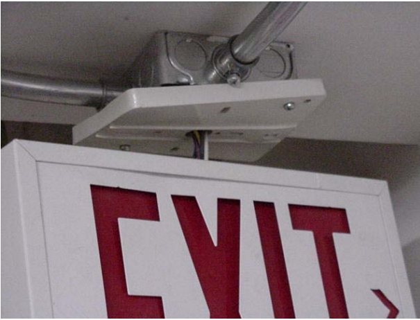
Exit sign in parkade is not securely fastened and is not illuminated.
