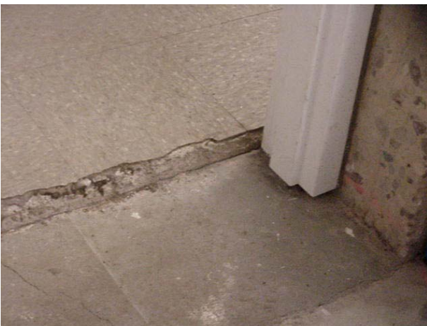
Step differential between parkade storeroom and hallway is a potential tripping hazard and should be graded.
