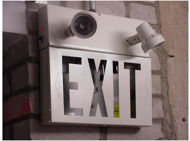
Exit sign in parkade is broken and not illuminated.
