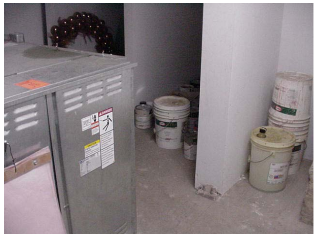
Storage of items in elevator machine room is in violation of the 1997 Fire Code and should be removed to a different location.
